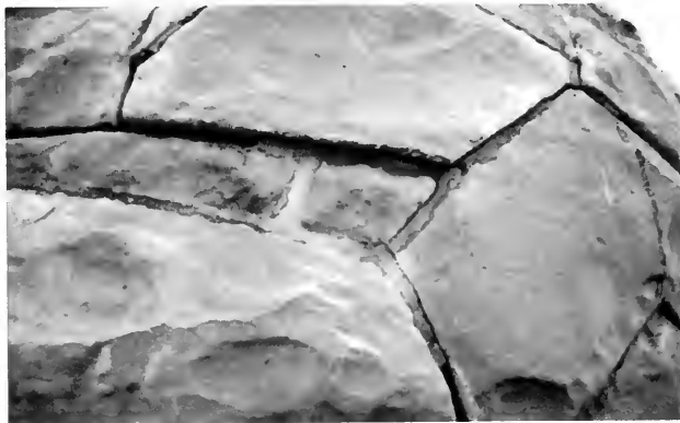
Figure 18: Inappropriate repointing of joints in rock mound base
